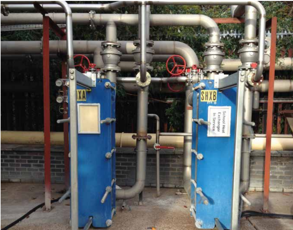
Standby heat exchangers at the North British Distillery in Edinburgh.
